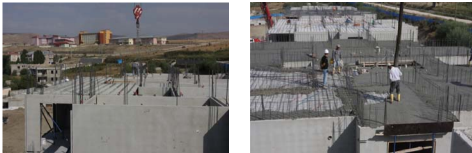
Fig. 1. Application of semi-precast slabs made of precast lattice girder planks and in-situ topping.
