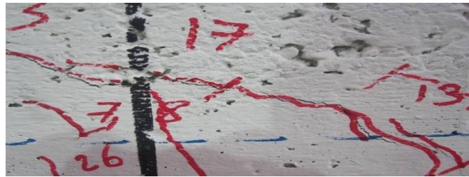
Fig. 5. Crack width in concrete and HPFRCC in RCH-0.2
