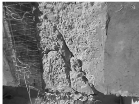
(e) Debonding of end anchorage due to shear failure of concrete
