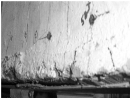
(c) Debonding in flexure zone
