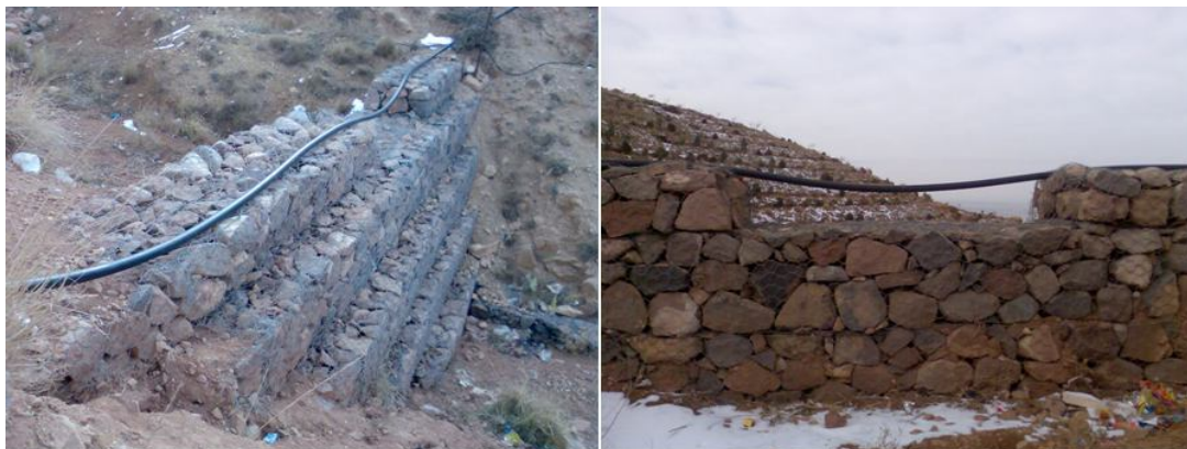
Fig. 1. Gabion stepped spillway used to reduce water velocity and to collect sediments in mountain valley (left), and gabion structure in a retaining wall for slope stability (right) on Onebne-Ali mountain, north of Tabriz (IRAN)
