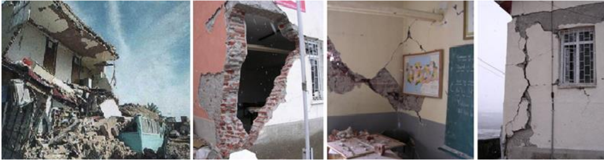
Fig. 1. Damage to masonry structures
