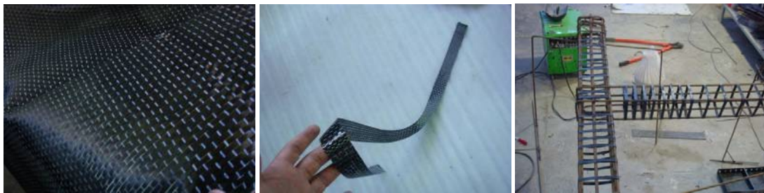
(a) Original FRP sheet (b) Cutting FRP strips (c) Stirrups installed in joints
