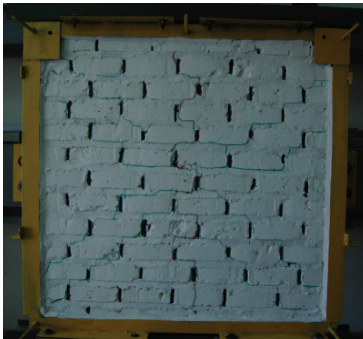
Fig. 20. Mode of failure of the wall NWEB
